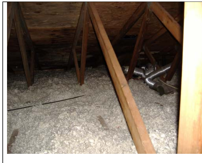
Discoloration, possible damage.
